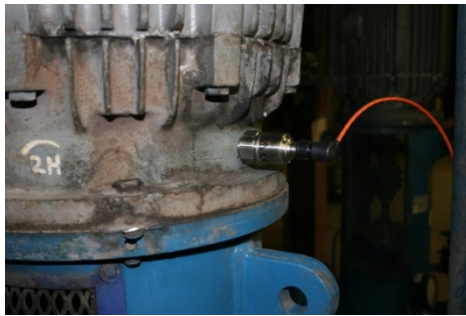
Figure 9: Permanently mounted ICP® accelerometer on a motor.
