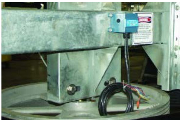
Figure 5 Mechanical Vibration Switch installed on a Cooling Tower Fan
