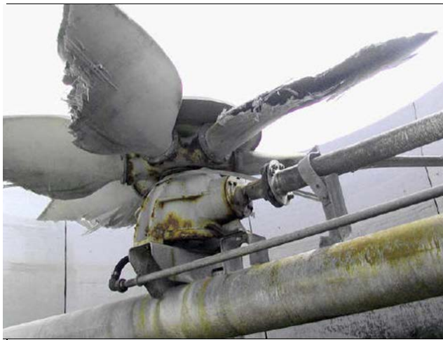
Figure 3(a) A failed Cooling Tower Fan
