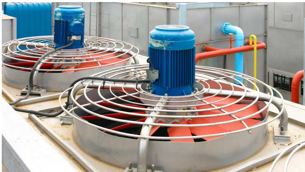
Figure 8 Electronic Vibration Switch mounted on a Cooling Tower Motor
